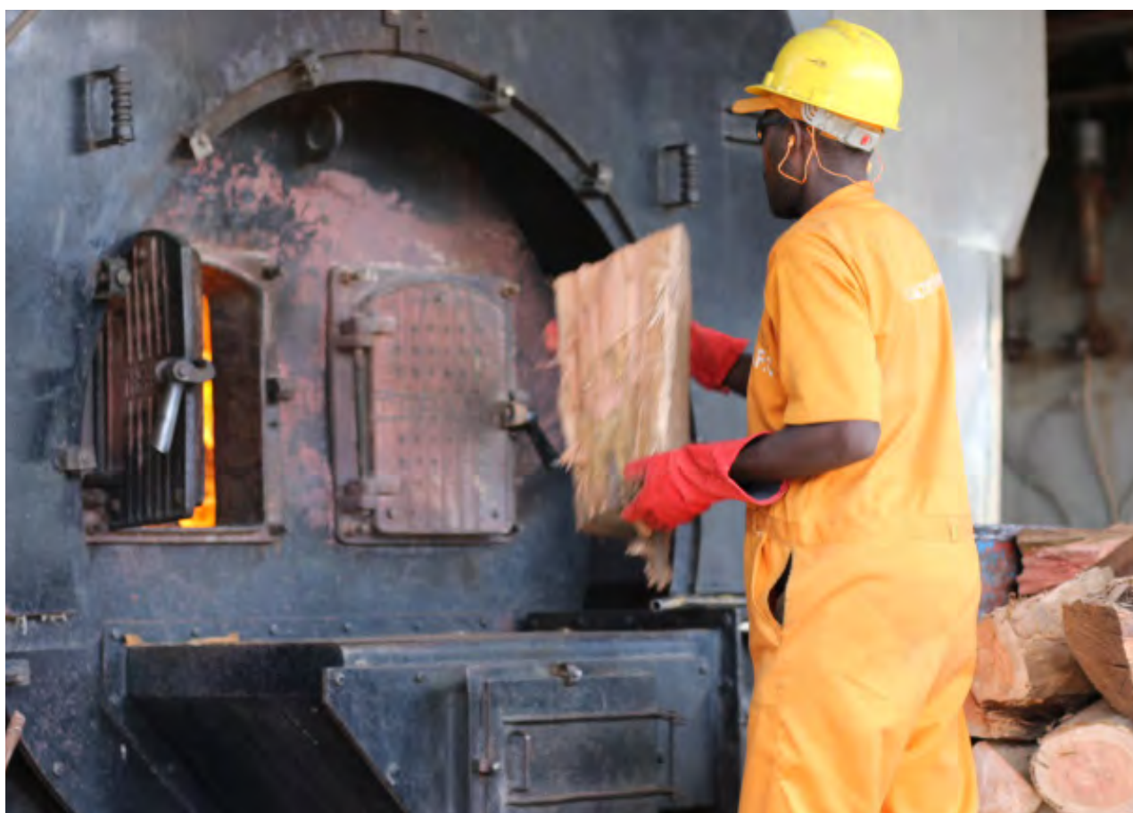
A worker loads firewood into the boiler at Mulindi factory
